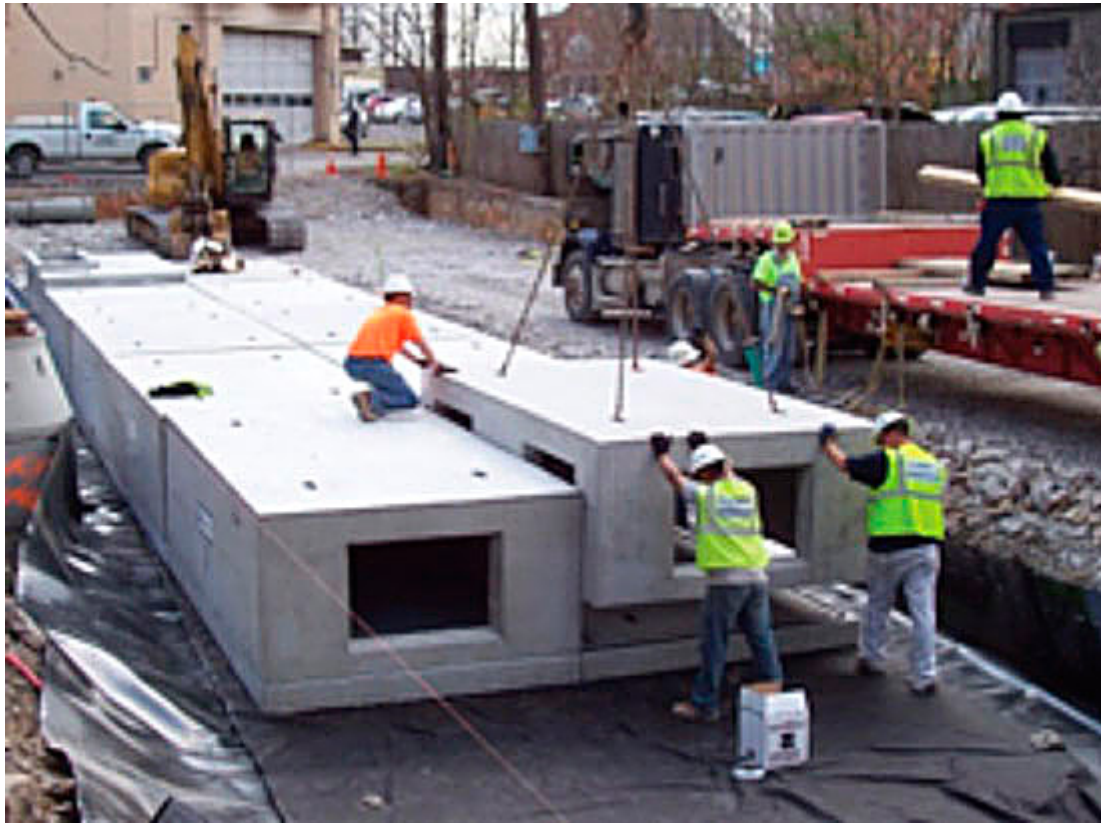
Figure 3: The Government of Nashville and Davidson County elected to remove an above-ground detention pond and construct an underground stormwater detention vault.
